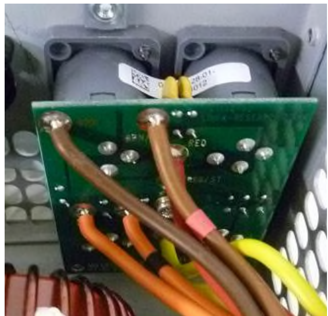
Wiring at rear of speaker connectors
